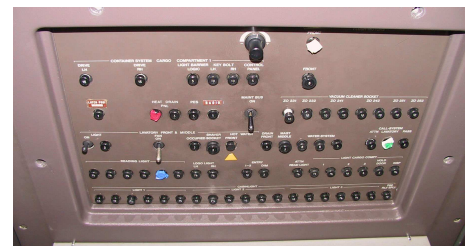
(a) Circuit Breaker Panel
